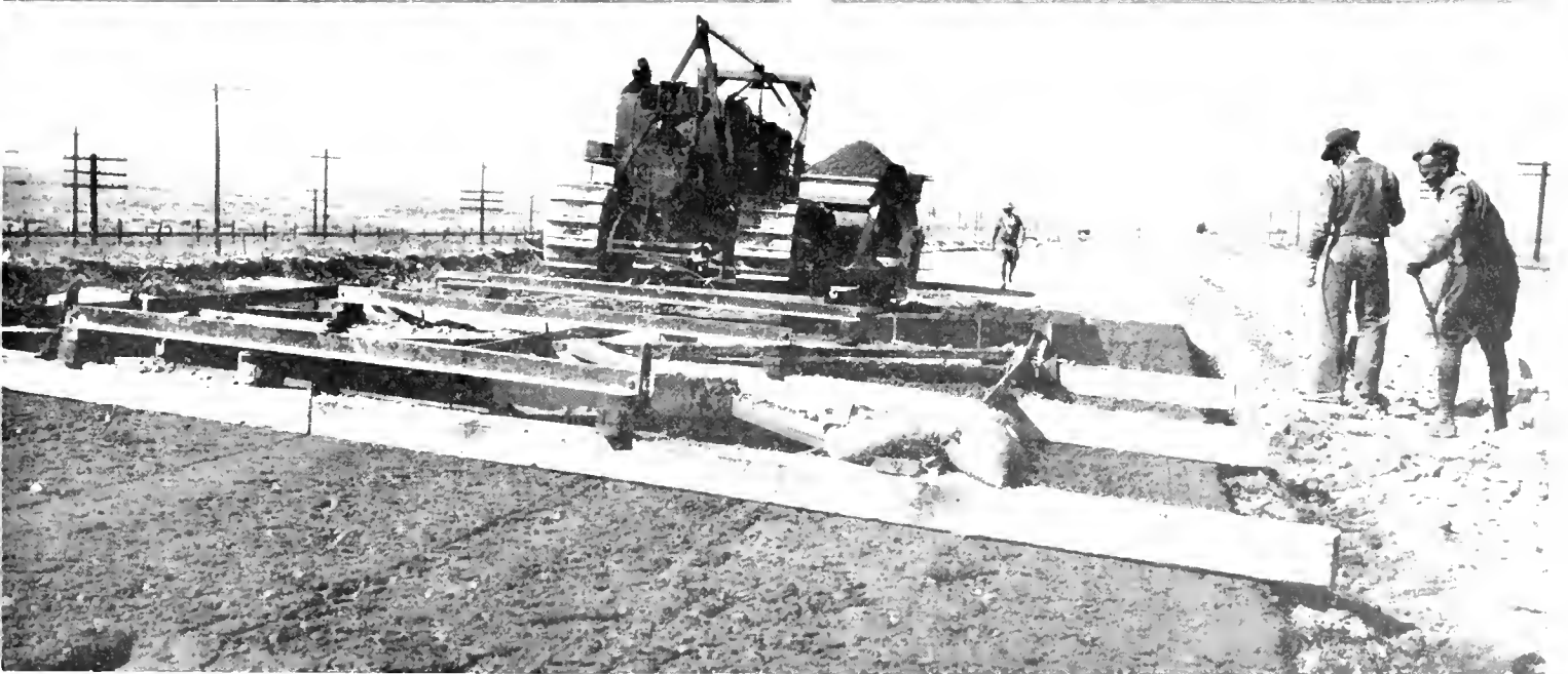
At top. One way traffic channels separate Indio and Palm Springs traffic at junction point. Overhead structure at left carries Palm Springs northbound traffic. Center. Section of new one-way road-bed. Existing roadway on left. Bottom. Spreading cement stabilized base. Bulldozer pushes laden truck, spreads material while dumping and pulls timber drag behind
